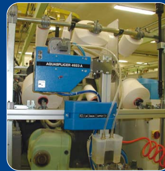
ATS "L" type with Aquasplicer 4923B fitted on slider for tail transfer at different level of fractional creel for cotton warping.
