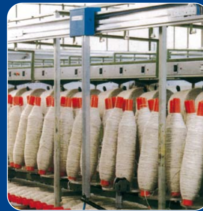
ATS "C" type installation with Jointair 116 on a carpet winder creel.
